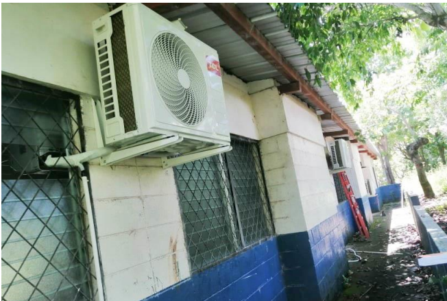
Air conditioners installed in Guajoyo School
