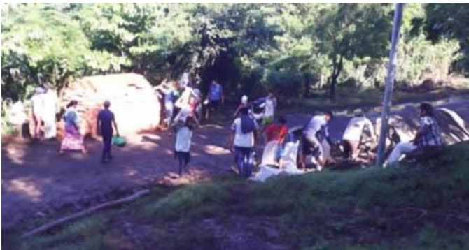
Volunteers from nearby Granzaso help move building materials from the road to the construction site
