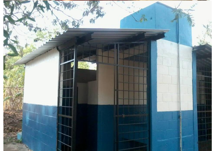
(Before and after photos of part of the Guajoyo School Lavatory Renovation)
